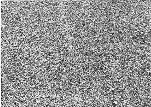
Additional seam wear and traffic-related surface deterioration.
